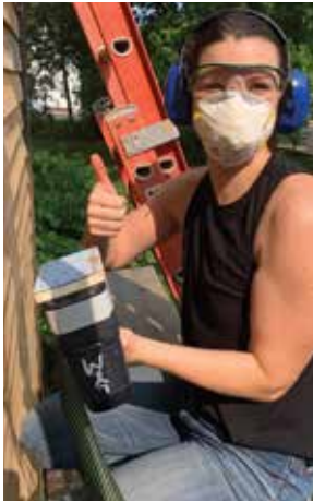
Left: Longyear volunteer sands wood clapboards in preparation for painting the Mary Baker Eddy Historic House in Amesbury, Massachusetts.
